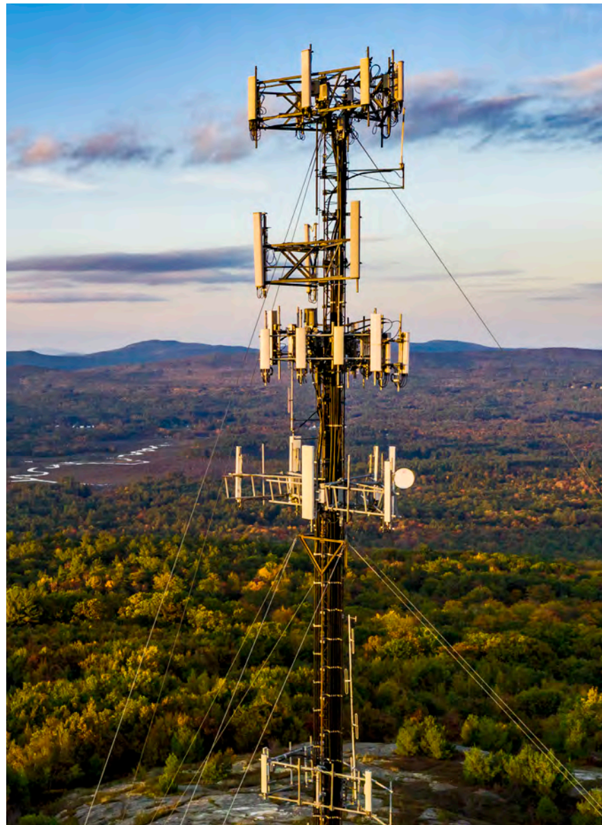
An American Tower wireless tower located in Needham, Massachusetts.
