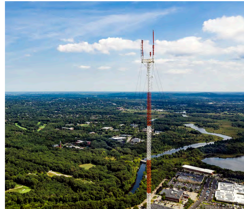
An American Tower wireless tower located in Alton, New Hampshire.
